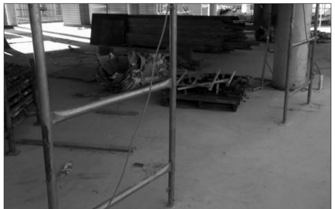
Kerry Vince Pty Ltd car park, offices etc site – poor housekeeping and leads contacting metal.
