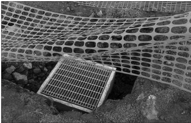
Unprotected drain hole in sports ground of the school. The ground is used at weekends for primary school sports. A young child fell down this hole injuring his leg. Wilkins Construction Pty Ltd St Alysios School Huntingfield.
