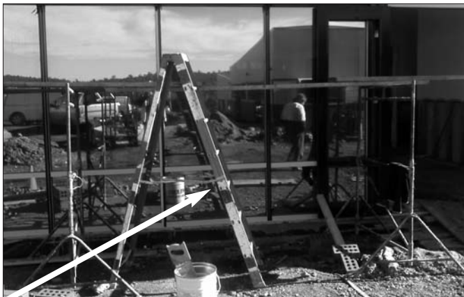
Unsafe scaffold lacking hand rails, erected on unstable muddy ground with a step ladder used as access. Wilkins Construction Pty Ltd site.
