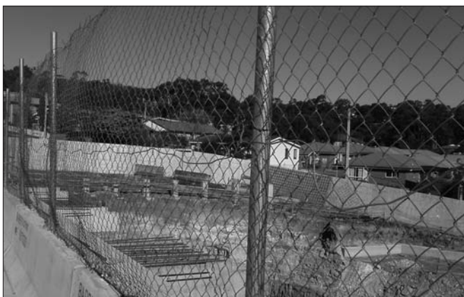
Apple Construction Pty Ltd shopping complex site – access area surrounding excavation lacking proper fall protection.
