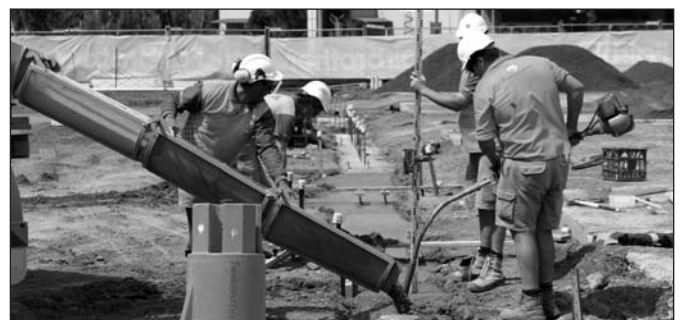
The new Coles supermarket at Mowbray in Launceston, on which Mick is foreman is due for completion in September. The Fairbrother team of about 7 workers were just finishing off the footings stage of the project when the Bluey visited on November 21. The 3700 square metre supermarket project will also create work for about 30 sub-contractors when the job gets going.
