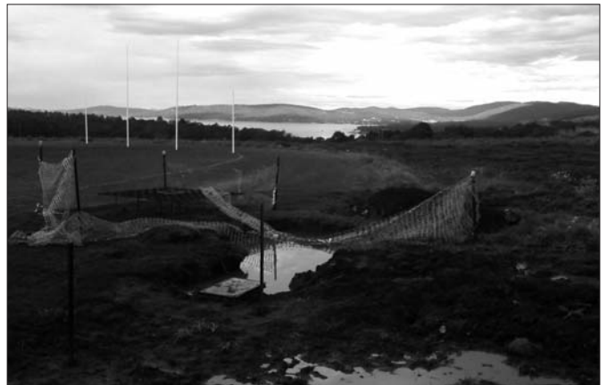
Same Wilkins Construction Pty Ltd site as photo 1, water about 1/2 meter deep – enough to drown a toddler.
